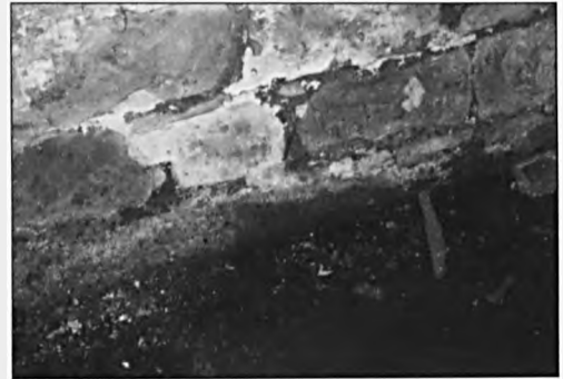
Fig. 16: Photograph showing the foundations of a stone wall in the cellars of Cambrian Road, Newport. (Copyright: Richard Frame).
