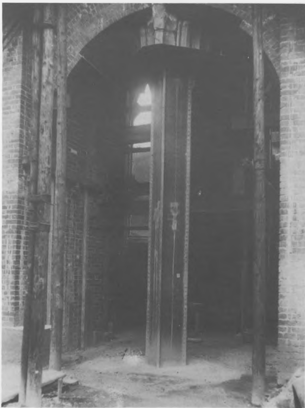
Plate 3: Office of Works — A view of one section of the south nave arcade during the 1920s conservation scheme. Brick supports have been raised and the masonry pier at the centre taken down. The steel stanchion has been put in place and awaits its cover of historic masonry (Cadw: Welsh Historic Monuments, Crown Copyright ).
