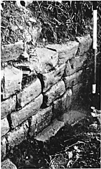
FIG. 4 The fortress-wall opposite the Amphitheatre, Caerleon, 1962. The original construction, with four courses of the facing, slab plinth, and traces of cobble foundation below.
